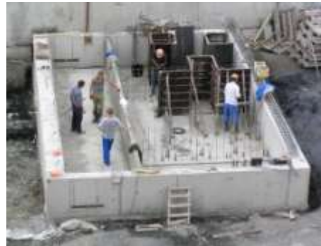
Transformer substation in the flood lands terrace of the Kacha-river
